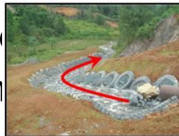
Drop Structure (WD4 RTU)
